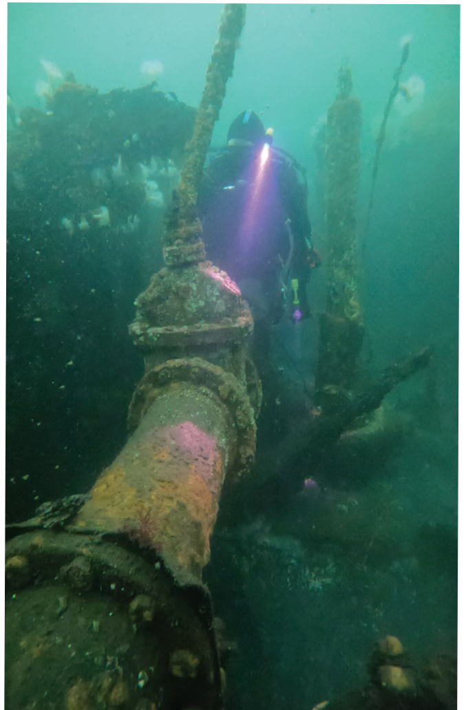
Paul Spencer examines large valve, part of the drydock pumping machinery.
